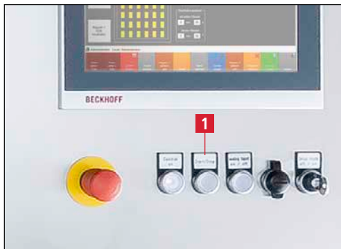
Figure 7-5 Control panel, grinding machine
