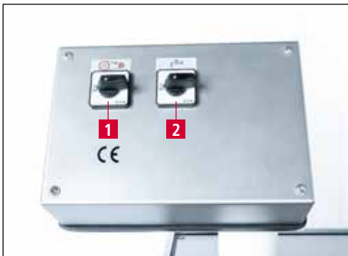
Figure 7-8 Control panel USK 230
